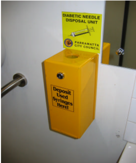
1.4 litre sharps bin installed within public toilet, Council Administration Building.
