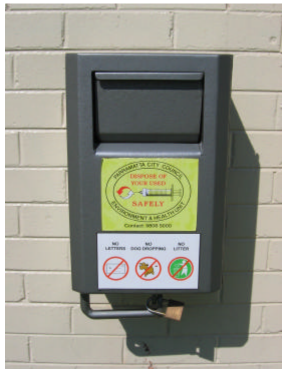
10 litre sharps bin installed on external wall, Jubilee Park Public Toilet, Parramatt
